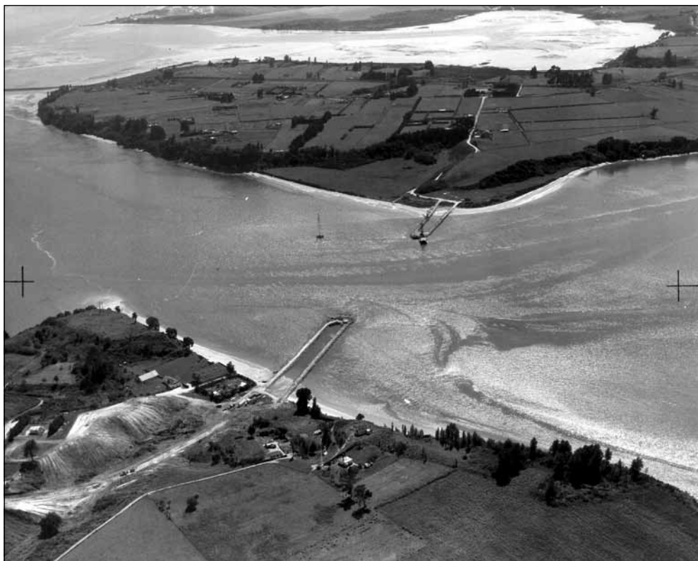
Figure 4.8: The Maungatapu Causeway under construction, 1958. Matapihi is top of photo, Maungatapu bottom foreground. Maungatapu Marae is on the shore, left of construction.
